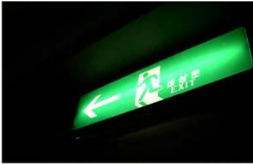
Instead of the entrance door use the emergency exit to evacuate
